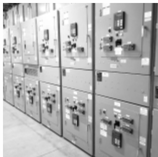
ELECTRICAL & SWITCH GEAR
